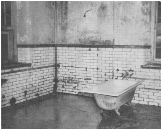
The bathroom in Female Ward 4. It is not possible in a photograph to recapture the squalor of this and other bathrooms in the Female section at Callan Park
